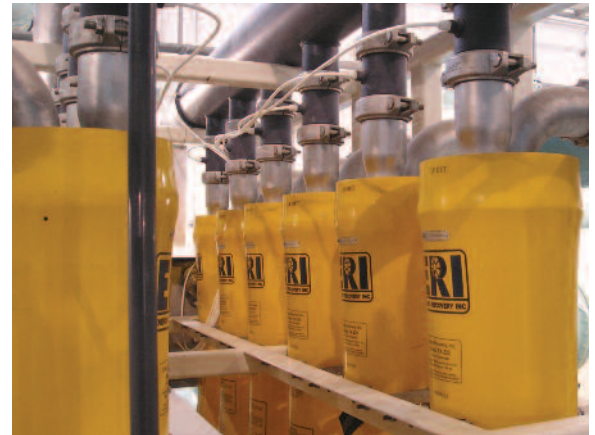
YuHuan Power Plant, China — Trains #1 and #2
