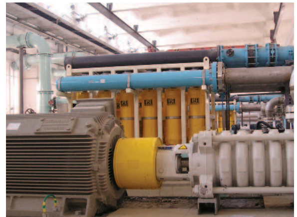
YuHuan Power Plant, China — Trains #1 and #2
