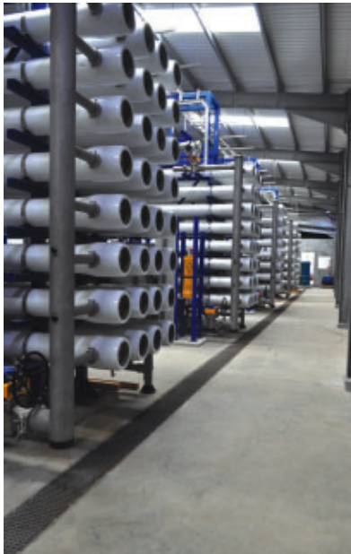
Inside the Biwater Tortola SWRO desalination plant
