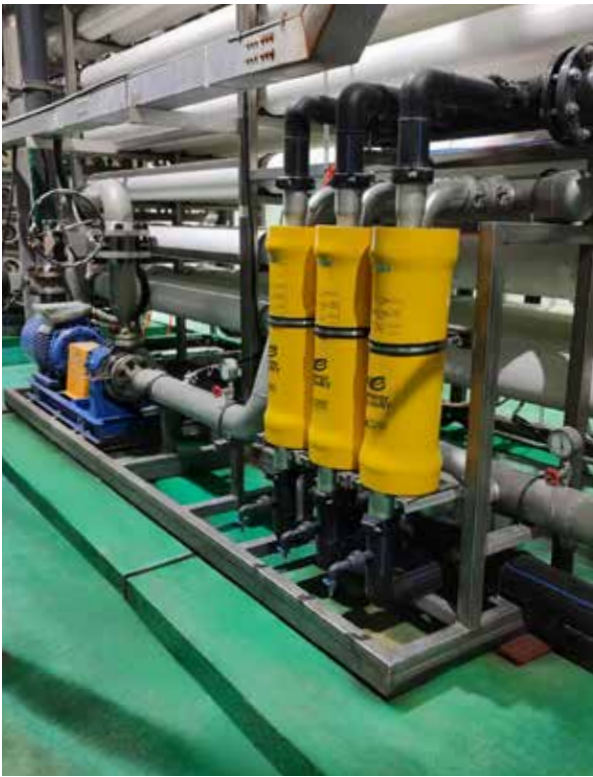
The facility also employs multiple PX Q260 energy recovery devices for energy reduction of their high-pressure flow streams.
